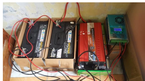
Figure 4 Battery, inverter and voltage stabilizer
